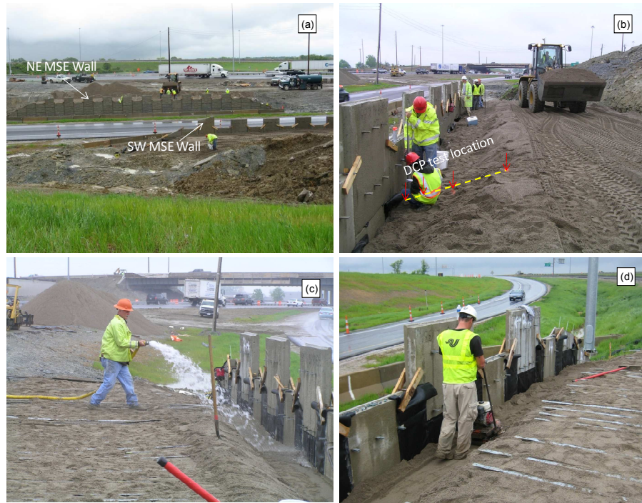
Figure 57. Bridge #1(BUT-75-0660) at I-75 &SR 129 interchange: (a) location of south and north MSE walls; (b) DCP test locations; (c) watering of backfill prior to compaction; (d) compaction of backfill next to the wall
