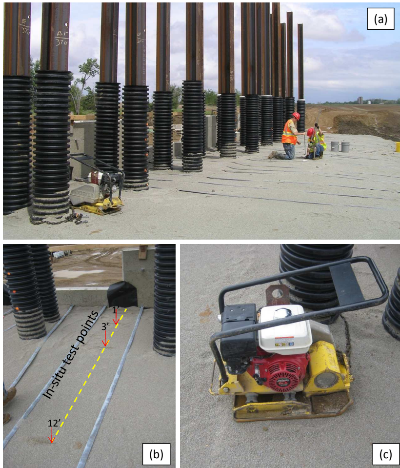
Figure 61. Bridge #2 at Wilmington: (a) overview of the south MSE wall; (b) DCP test locations; (c) vibratory plate compactor used to compaction of wall backfill
